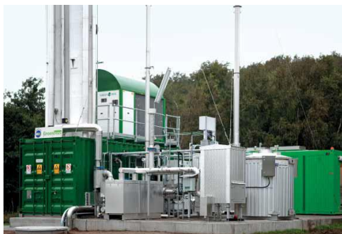
Figure 4 : The only Danish upgrading plant in Fredericia (Water Scrubbing)
