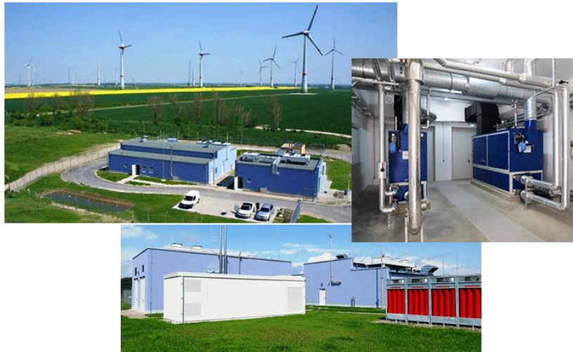
Figure. 6: Grapzow, Germany. 1 MW electrolyzing system (Hydrogenics) - 210 Nm 2 hydrogen/hour. Taking power from 140 MW wind farm.
