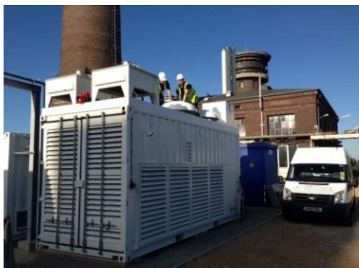
Figure 4: ITM - 315 kW PEM electrolyzer (60 m 3 Hydrogen/hour)
