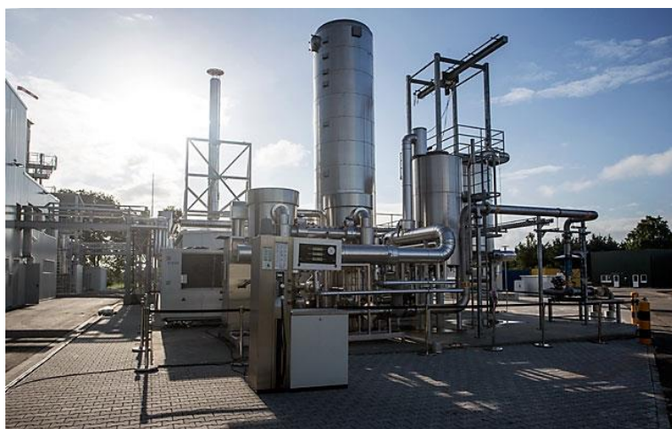
Figure 7: 6 MW Alkaline electrolyzer. 1300 Nm 3 hydrogen/hour (+ 300 Nm 3 SNG when methanization plant is established)
