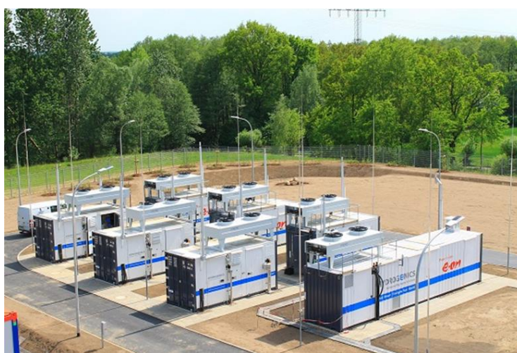
Figure 5: E.ON Falkenhagen, 2 MW alkaline electrolyzer plant.
