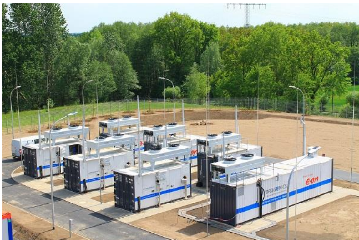
E.ON Falkenhagen 2 MW Alkaline electrolyzer (Hydrogenics). Start-up
